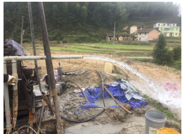
Figure 8. The ground water well at the 400 position.
